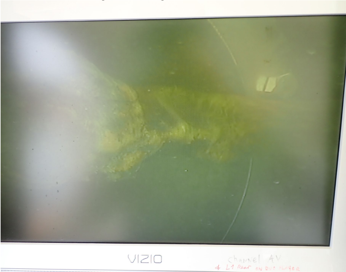
Picture 1: Underwater image of debris lodged in orifice 1A2.
